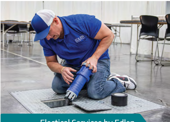
Electrical Services by Edlen
